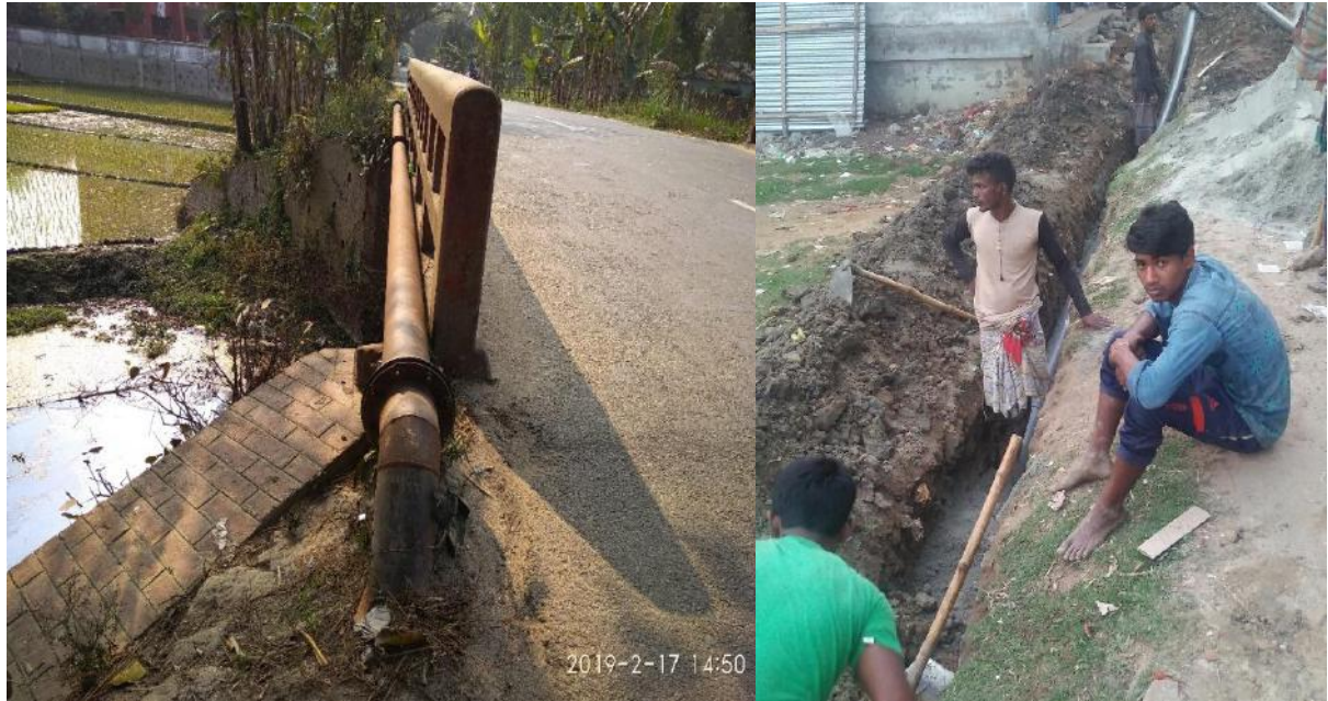
Figure 18 Existing and newly constructed pipelines in Bera
