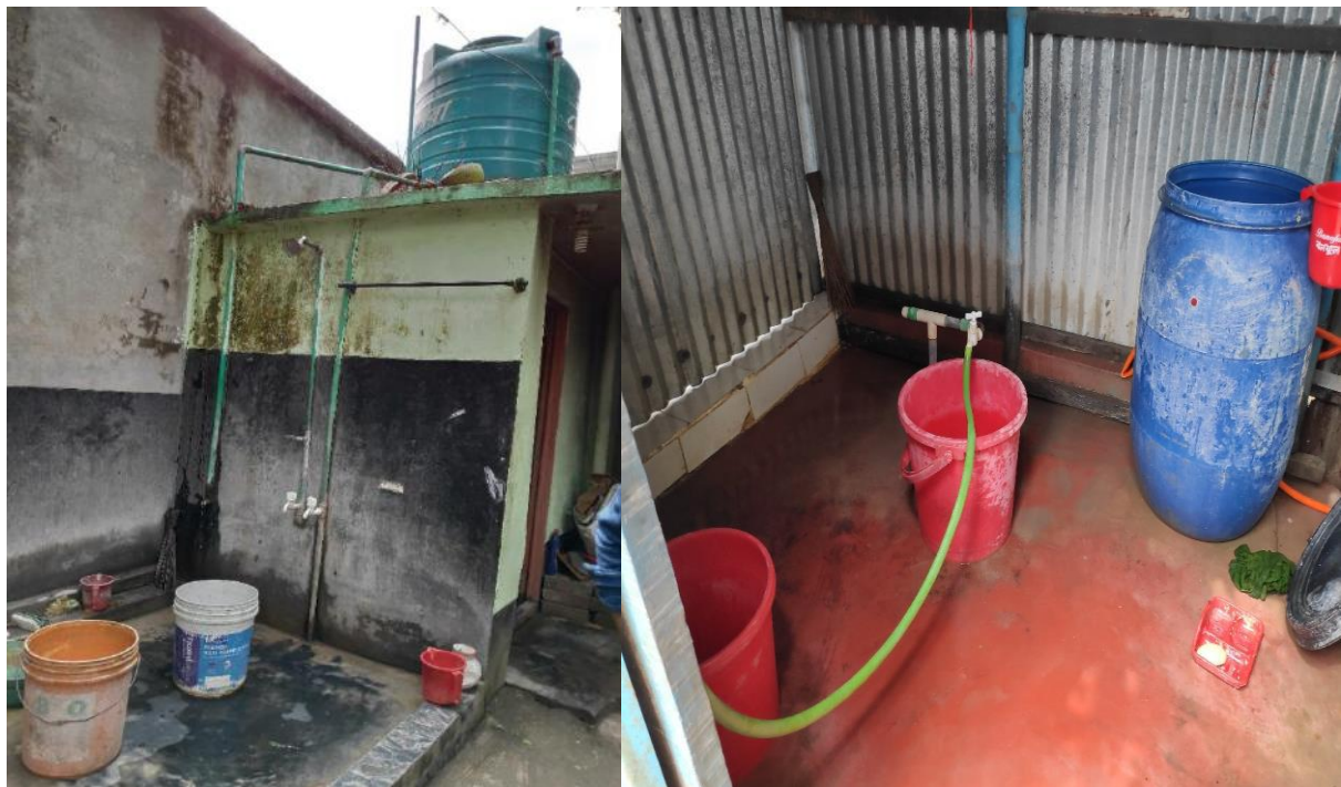
Figure 17 House connection in Jhikargacha
